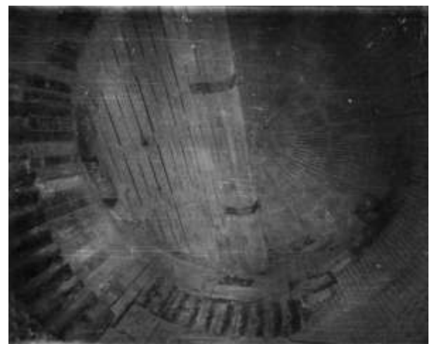
Fig. 10 Blade elliptical segment installed at the discharge bottom of the mill \varnothing 3.2 \times 15\text{ m}
